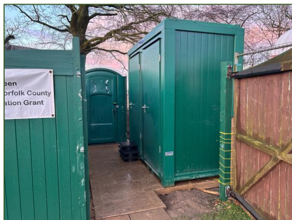
New toilet block and ladies toilet (temporary) installed in their final positions
